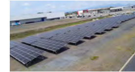
Solar power generation facilities (Nippon Cookery Co., Ltd., Isesaki plant)
