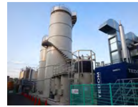
Biomass Electricity Generation at the Hachioji General Plant
