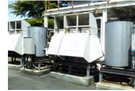
Chiller (Cooling water circulation equipment)
