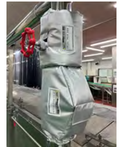
Improved Thermal Insulation Through the Use of Insulation Jackets
