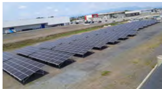
Solar Power Generation Facilities (Nippon Delica Service Co., Ltd., Isesaki Plant)
