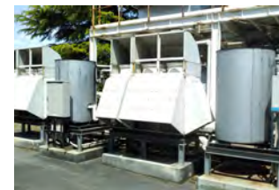
Chiller (Cooling Water Circulation Equipment)
