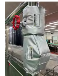
Improved Thermal Insulation Through the Use of Insulation Jackets
