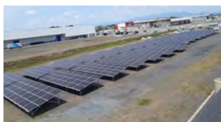
Solar Power Generation Facilities (Nippon Delica Service Co., Ltd., Iseaki Plant)
