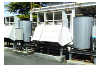
Chiller (Cooling Water Circulation Equipment)
