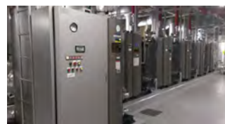
Fish Oil-Fueled Boiler (Fine Chemicals General Plant Kashima No.1 Plant)
